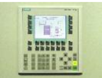
Through a tableau with a display and keyboard all processes for the crane, dryer and gasifier are controlled.
